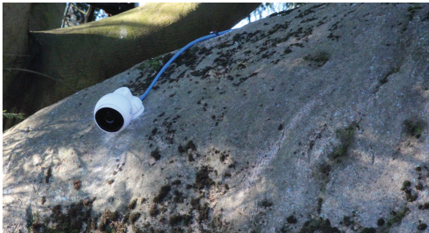
UniFi camera installation
