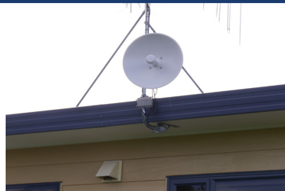
ePMP Force 200 connecting a residence
